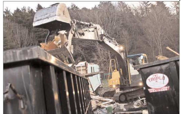
Workers from Gene Armstrong Excavating remove the damaged mobile homes from Glen Park in West Brattleboro. (Zachary P. Stephens/ Brattleboro Reformer)
